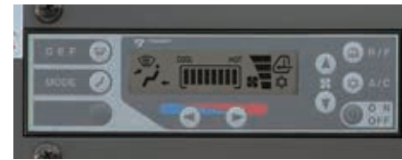
Air conditioner Hot-water heater and air conditioning.
